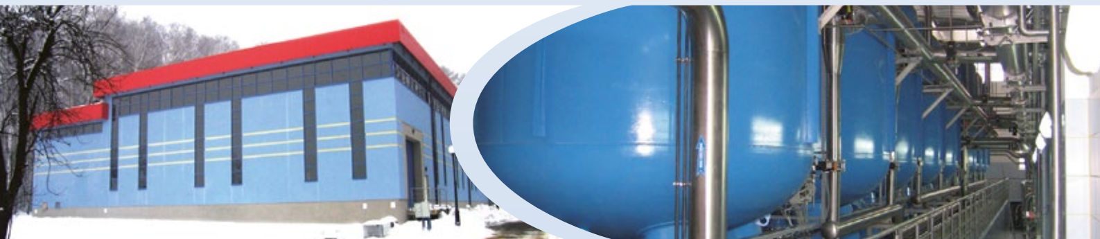
Czestochowa, Poland Commissioning 2006, 12'000 m 3 /d
