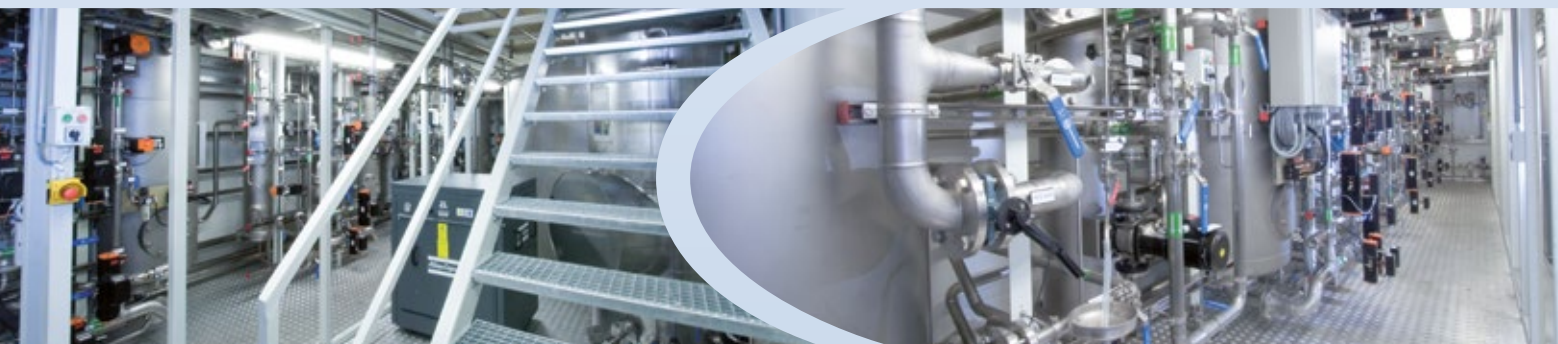
BIODEN® Containerised testing plant Commissioning 2007, 100 m³/d
