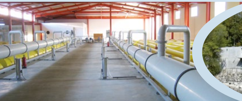
Benalmádena WWTP, Spain BIOPUR®-C and disinfection for water reuse (irrigation) Commissioning 2007, 273'000 p.e.
