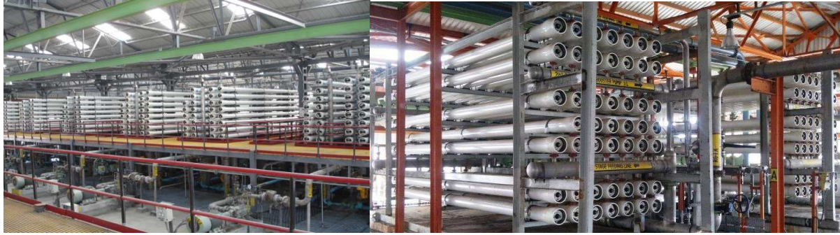
Figure 4 PRE-WRP and RE-WRP - reverse osmosis systems
