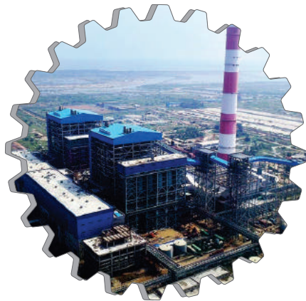
Complete water system for 2x800 MW Supercritical Thermal Power Plant at Krishnapatnam, Nellore district, Andhra Pradesh
