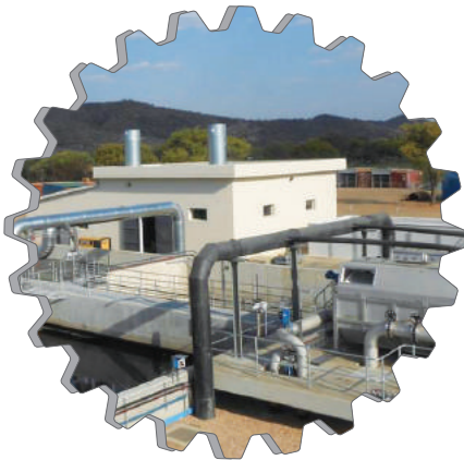
Industrial Park Ujams, Windhoek. First industrial Reuse & Wastewater MBR plant in Namibia. Capacity : 5,175 m 3 /d
