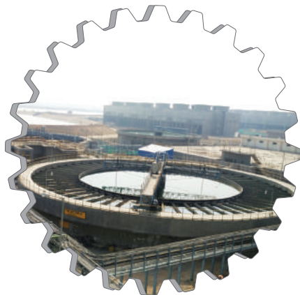
Power plant water system (pretreatment, RO-DM, SSF, chlorination system) India
