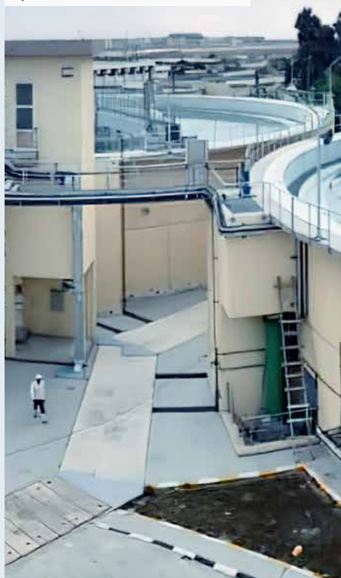
El Raswa WTP II, Port Said, Egypt: multi-stage system for treatment of Nile water, 80,000 m 3 /d
