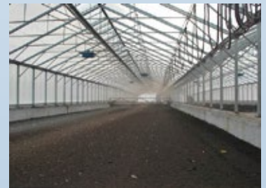
Solar sludge drying
