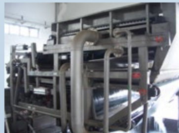
Sludge dewatering (belt filter press)
