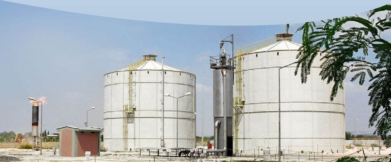
Biogas desulphurisation, gas storage, excess gas burning (Adana West WWTP, Turkey, 250,000 m³/d)
